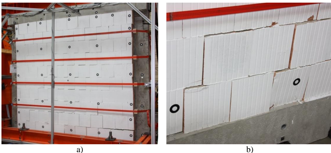
Figure 5.39 a) Diagonal cracks in the wall and b) opening of bed joints
