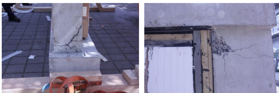
Figure 5.85 Cracked frame at the end of the test
