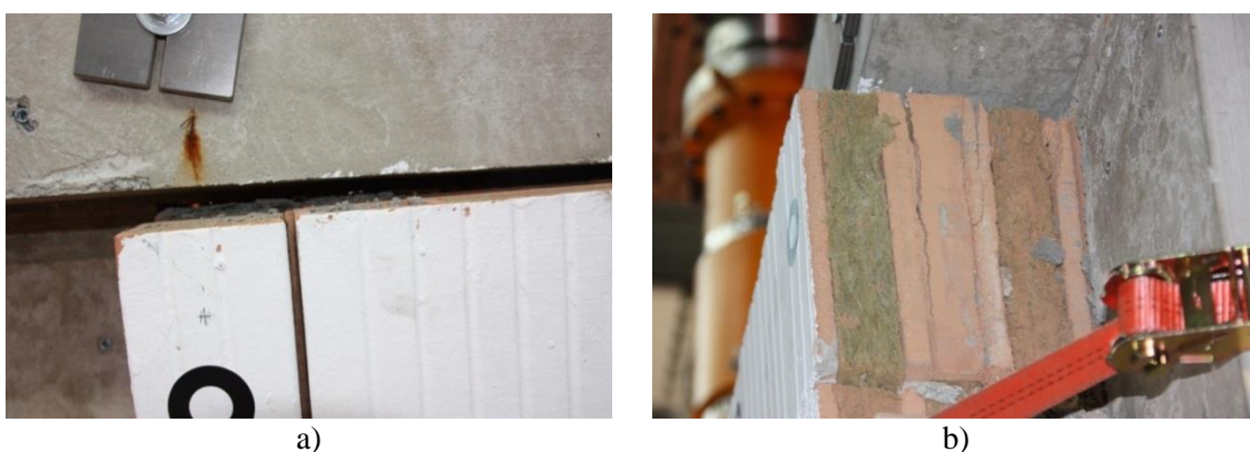
Figure 5.36 a) Damaged mortar connection between infill wall and concrete beam and b) splitting of the brick
