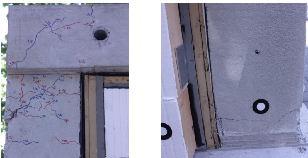
Figure 5.88 Cracks in the frame at the end of the DIO test
