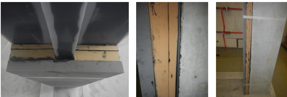
Figure 3.8 Placing U-shaped elastomers at the columns and top beam of the RC frame
