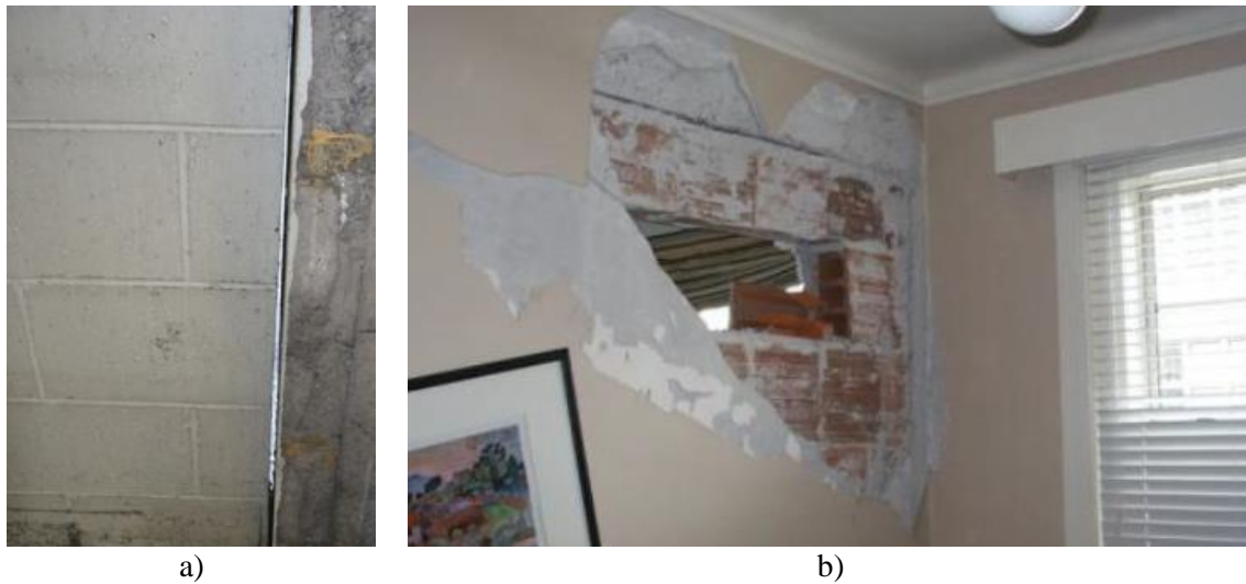
Figure 1.8 a) Separation of infill wall from the frame and b) corner crushing with the overall corner damage (Tasligedik, 2014)
